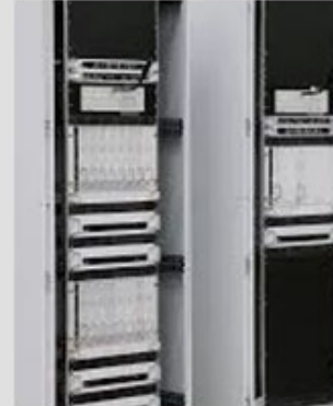
PA/GA NETWORK SYSTEM
