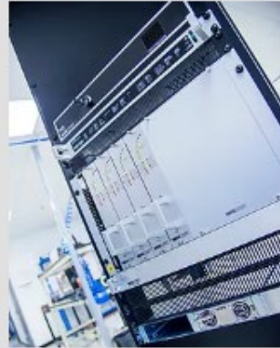
CEAS STANDALONE PA/GA SYSTEM
