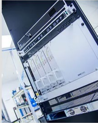
CEAS STANDALONE PA/GA SYSTEM
