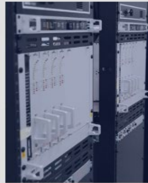
PA/GA NETWORK SYSTEM
