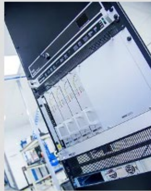
CEAS STANDALONE PA/GA SYSTEM
